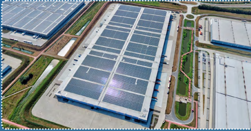
Solar panels and battery storage Lidl Venlo
