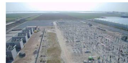
MS-MS station (3-23kV)
